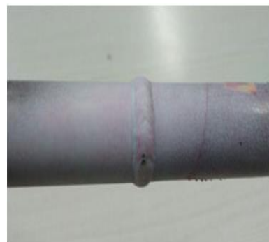
Figure 8. Inspecting of defect after DP test
